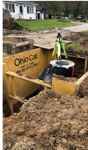
GPS Surveying equipment is used to ensure accurate locations and elevations of all pipes and manholes
