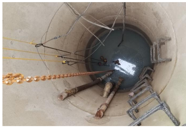
The inside of the pump station as seen to the left. Visible in this photo are two discharge force mains, chain for pump removal, access steps, and pump control equipment.
