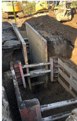
Trench boxes are used to protect workers against cave ins while laying pipes and setting manholes
