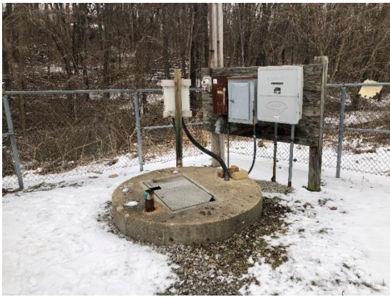
The exterior of one of the nine sewage pump stations in the Smithfield Wastewater System
