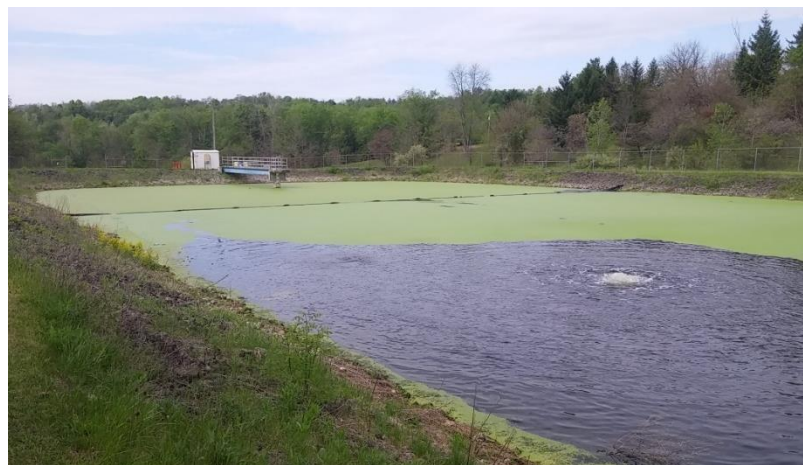
One of the two aerated lagoons located at the Smithfield Wastewater Treatment Plant. These lagoons create an aerobic environment which promotes the natural breakdown of wastewater solids.
