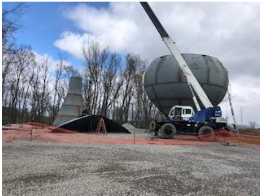
Various custom pieces of metal were shipped to the site, where they were then welded together to create the new tank bowl and tank base.
