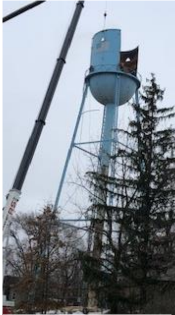
Demolition of the old Smithfield Water Tank took place in December of 2019.
