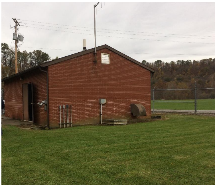
The Reeds Mills Pump Station Site will soon include a new building to house the electrical systems needed to keep this pump station running 24/7.
