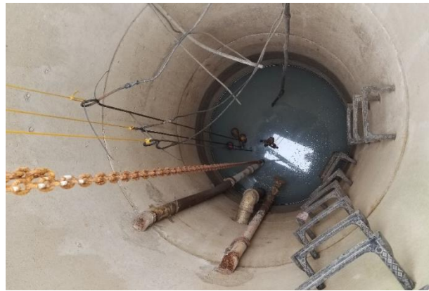
The inside of the pump station as seen to the left. Visible in this photo are two discharge force mains, chains for pump removal, access steps, and pump control equipment.
