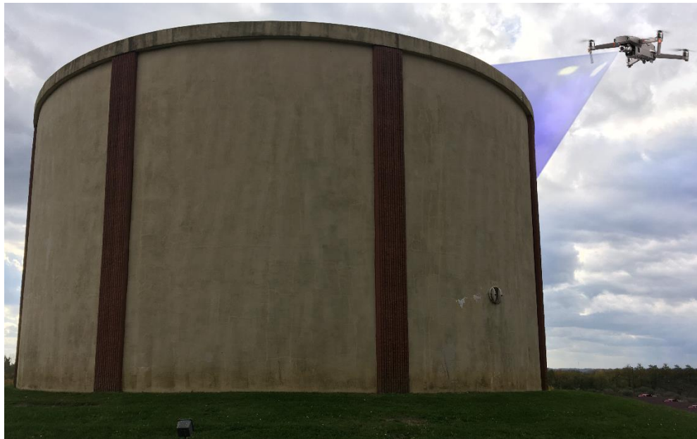
A mockup of a drone inspection of the Norton Hill Tank, which sits next to the Jefferson County Water and Sewer District's Service Center headquarters.
