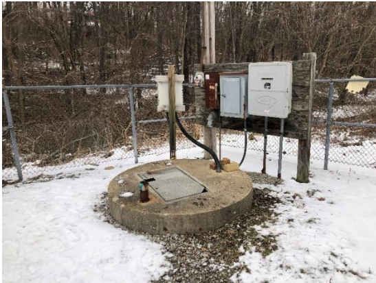
The exterior of one of the nine sewage pump stations in the Smithfield Wastewater System
